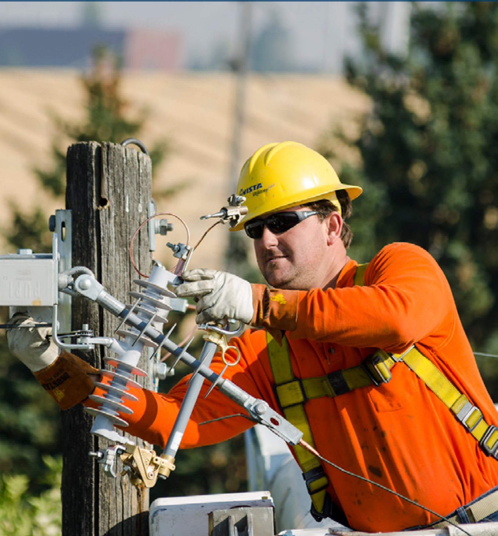
An Avista lineman upgrades pole components to support Avista's grid modernization program
